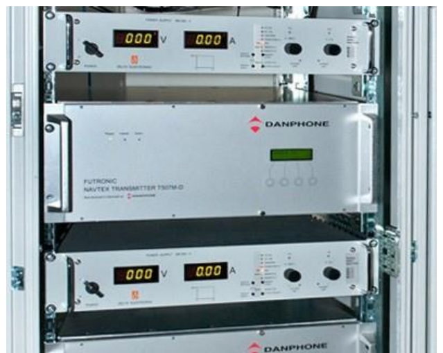
DANPHONE'S NAVTEX TRANSMITTER SYSTEM
