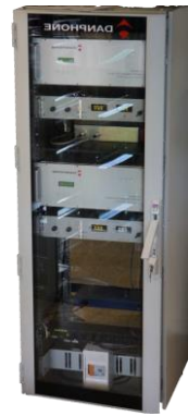
NAVTEX rack with two redundant transmitters
