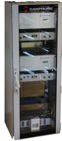
NAVTEX rack with two redundant transmitters
